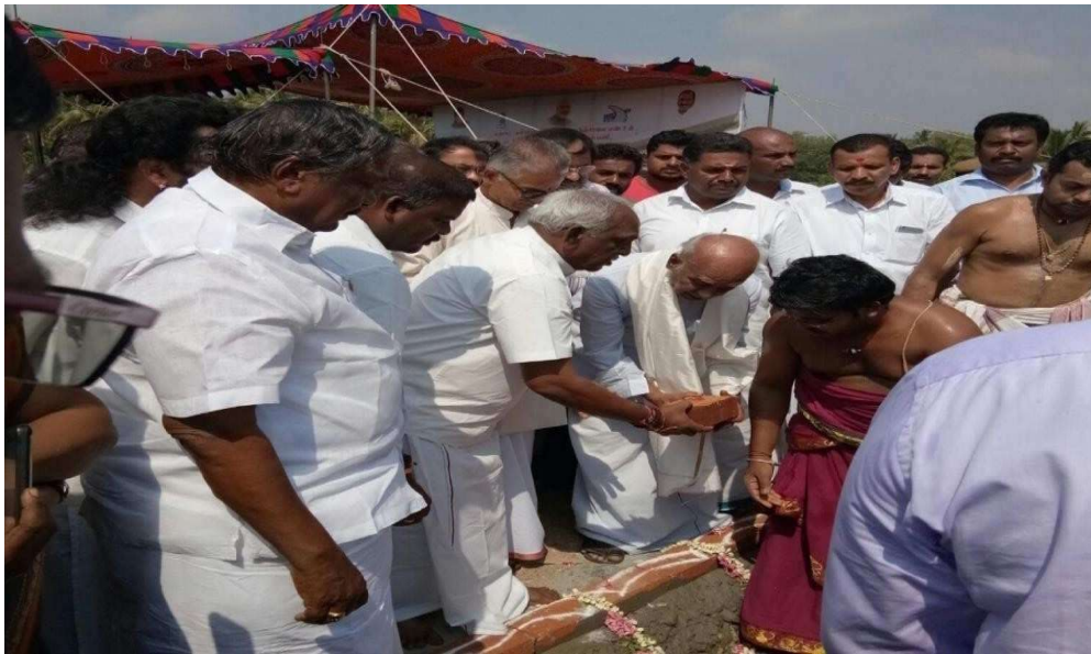
FOUNDATION STONE POOJA IN NARIKULAM TANK BY THE HON'BLE MINISTER OF STATE FOR ROAD TRANSPORT & HIGHWAYS FOR CONSTRUCTION OF 4 LANE ROAD AT MADURAI - KANYAKUMARI SECTION OF NH44 (OLD NH-7) IN THE STATE OF TAMIL NADU
