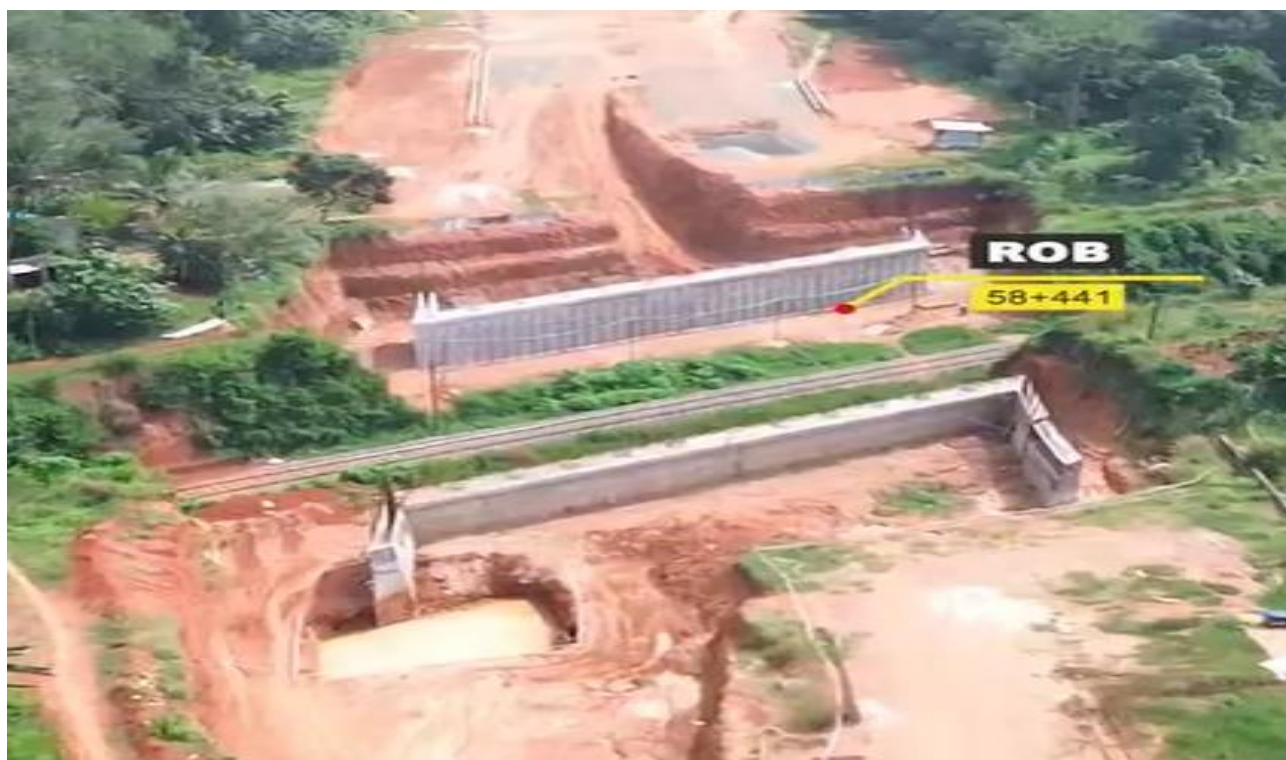
Four laning of Left-over works including additional structures in Kerala / Tamil Nadu Border – Kanyakumari from Km.43/000 to Km.96/714 of NH 47
