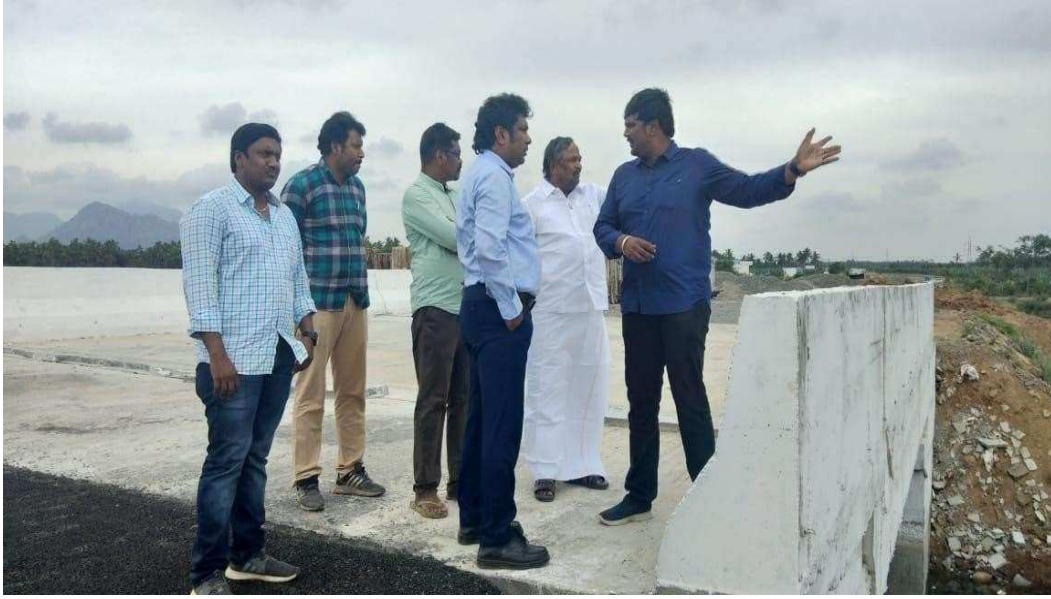
Narikulam Tank Construction at Madurai - Kanyakumari section of NH44 (Old NH-7) in the state of Tamil Nadu
